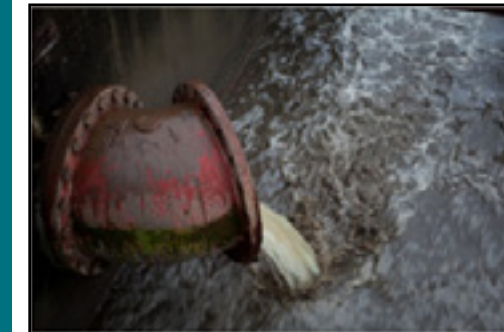
A wastewater treatment discharge point.
